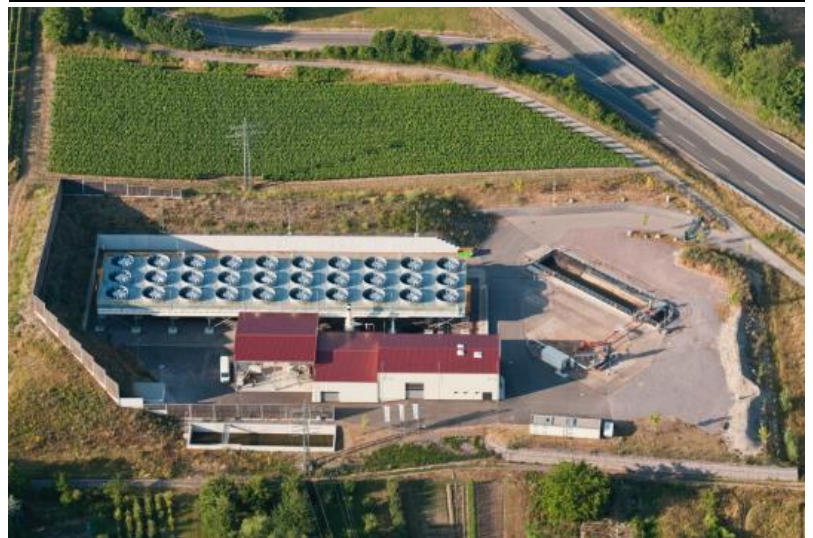
Figure 5: Vulcan has acquired the Insheim geothermal plant in Germany. The plant has 4.8MW of capacity and was EBITDA positive in CY20
